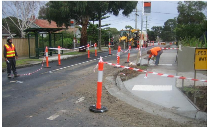
Bayside's commitment to green purchasing has resulting in significant use of recycled concrete in roadworks.
