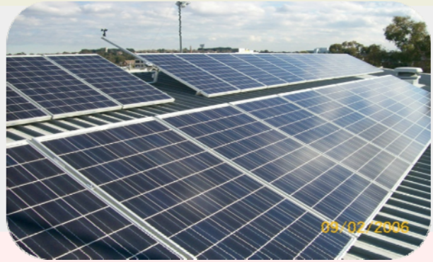
7.6kW solar PV System on Box Hill Town Hall
